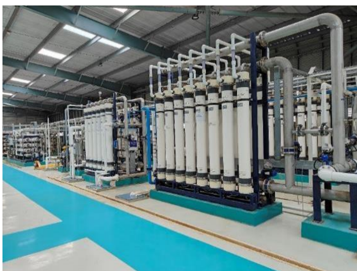
Ultra-pure water generation plant at Unit II
